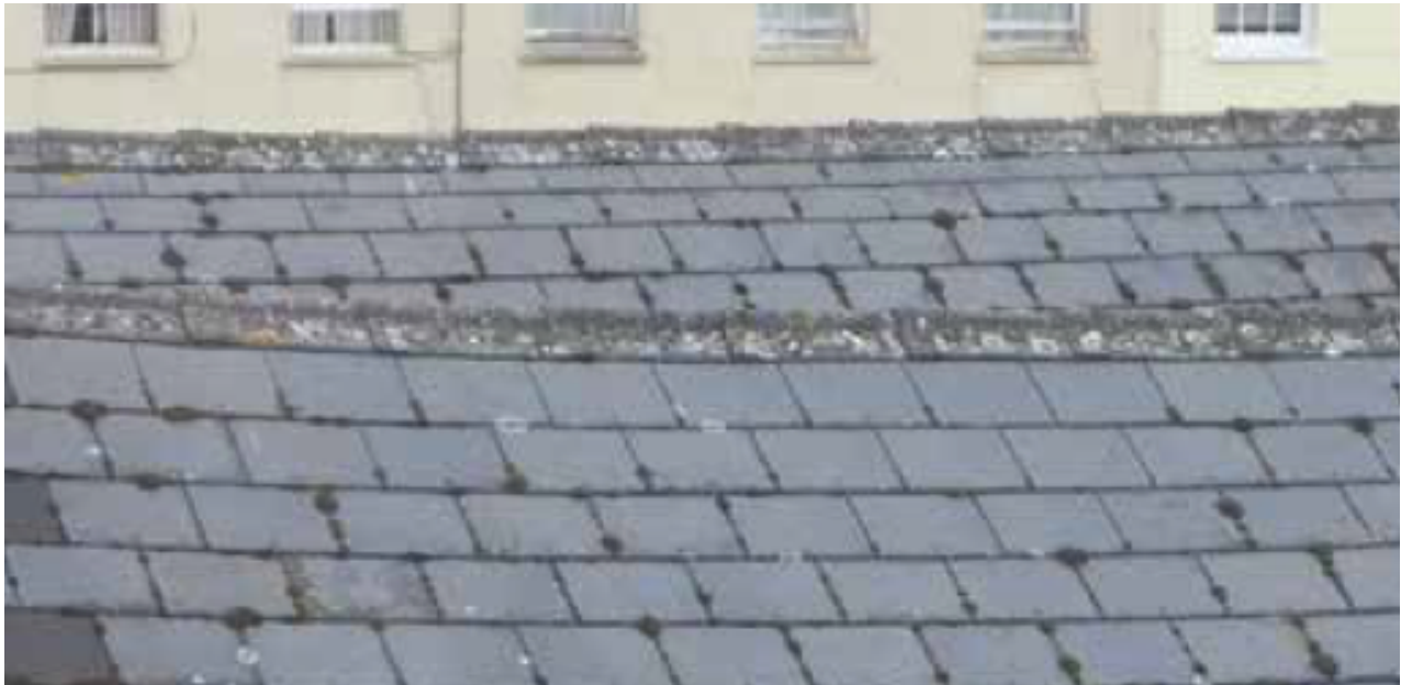
Two adjacent pitched roofs. The sag to the roof in the foreground could indicate a defect with the supporting structure beneath.
